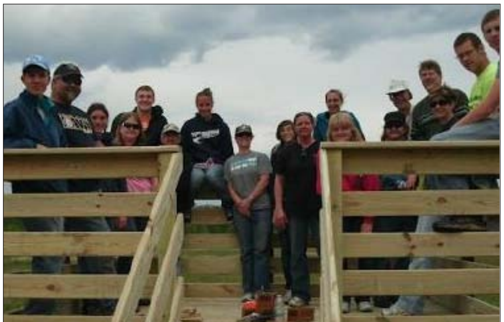
Grace Church's volunteers built a new viewing platform as a practice run for their trip to Appalachia.
